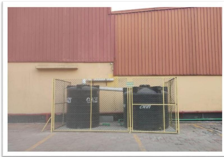
Figure: Rain Water Harvesting Tank
