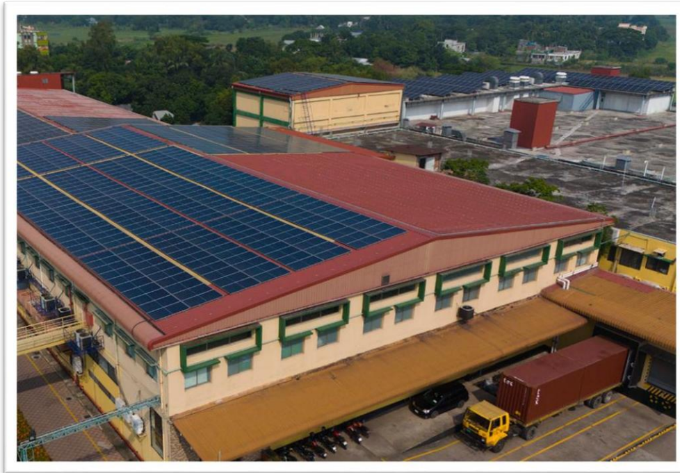
Figure: Solar Panel Installed in DBPL Rooftop
